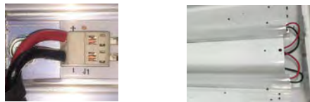
Installing LED Strips in Fixture With TEK Screws, Connecting power lines, replacing Ballast cover and install snap-on diffusers
